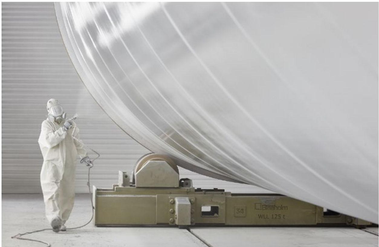
Application of surface protection on tower segment of wind power station in Give, Denmark
